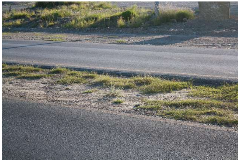
Grass and loose gravel occur in median at Tierra Soberana Blvd.
