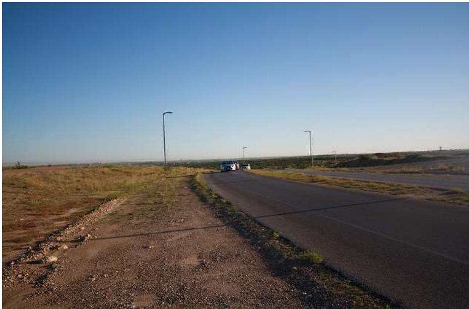
Curves without signage & gravel shoulders on Tierra Soberana Blvd.
