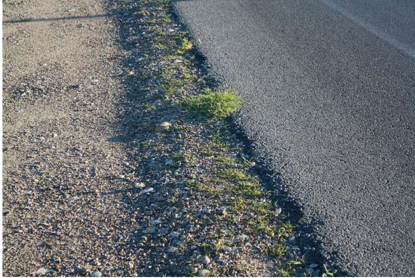
Loose gravel on crumbling shoulder at Tierra Soberana Blvd.
